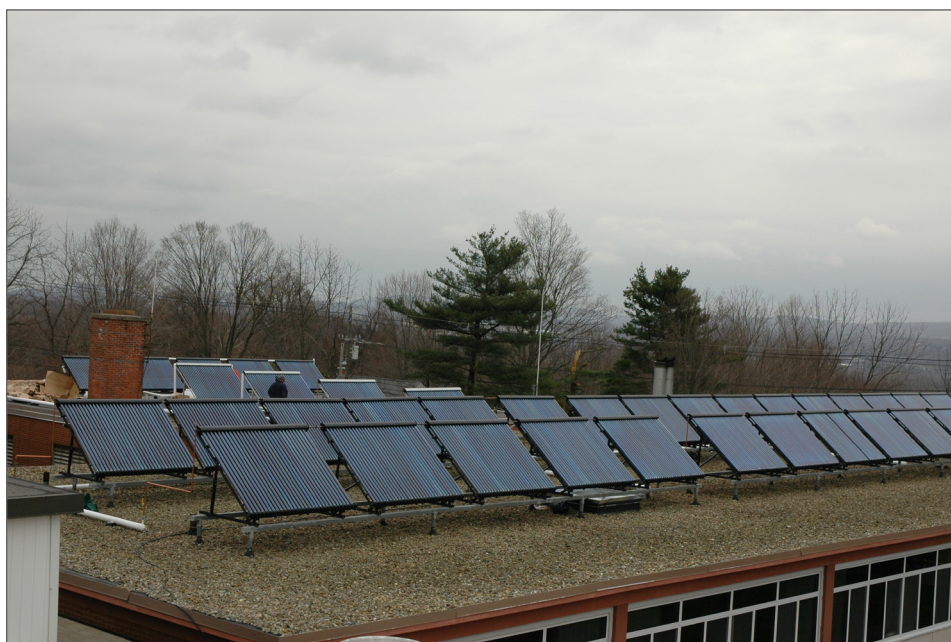
Solar water heating panels on the Gaylord hospital in Wallingford, CT
